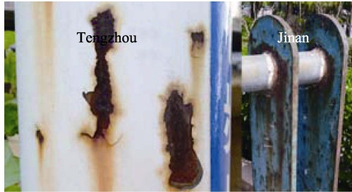
图 5 枣庄滕州和济南街道上碳钢结构涂层破损情况 Fig.5 Coating damage of carbon steel structures in streets of Tengzhou of Zaozhuang and Ji'nan
