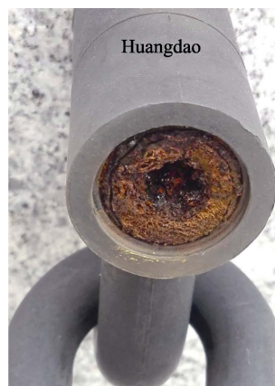
图 9 青岛黄岛区海滨景观碳钢锁链的塑料管包覆防腐 Fig.9 Plastic pipe cover anticorrosion for carbon steel chain in Seaside Landscape of Huangdao District, Qingdao
