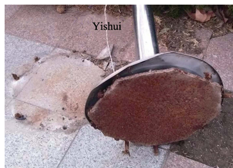
图 14 临沂沂水街道的一不锈钢结构因碳钢螺栓完全腐蚀而倒伏 Fig.14 A lodged stainless steel structure in street of Yishui, Linyi due to fully corrosion of carbon steel bolts
