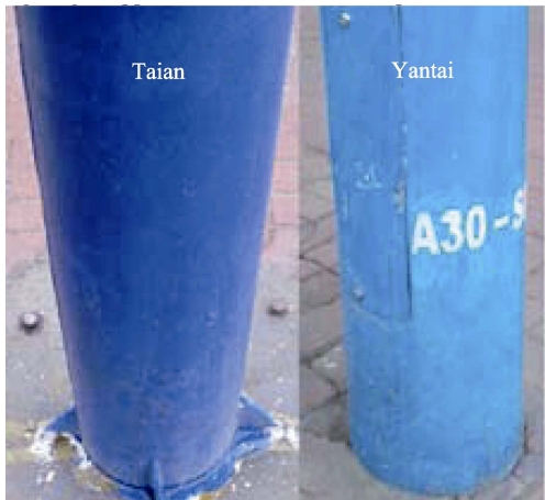
图 4 泰安和烟台街道上普通油漆涂装的街道照明灯柱 Fig.4 Street lighting lampost coated with aluminum paint in Tai'an and Yantai
