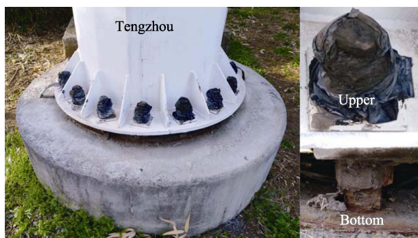
图 13 枣庄滕州某信号塔底座地脚螺栓腐蚀防护情况 Fig.13 Corrosion protection for the anchor bolts of a signal tower in Tengzhou of Zaozhuang
