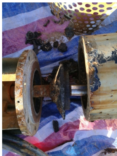
图3 油料装备排气管道高温腐蚀 Fig.3 High temperature corrosion of oil equipment exhaust pipe
