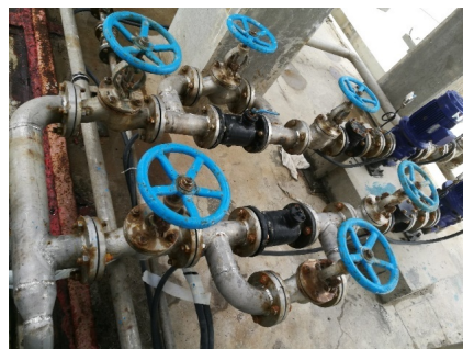
图2 油料管线及阀门(电偶腐蚀) Fig.2 Oil pipeline and valve (galvanic corrosion)
