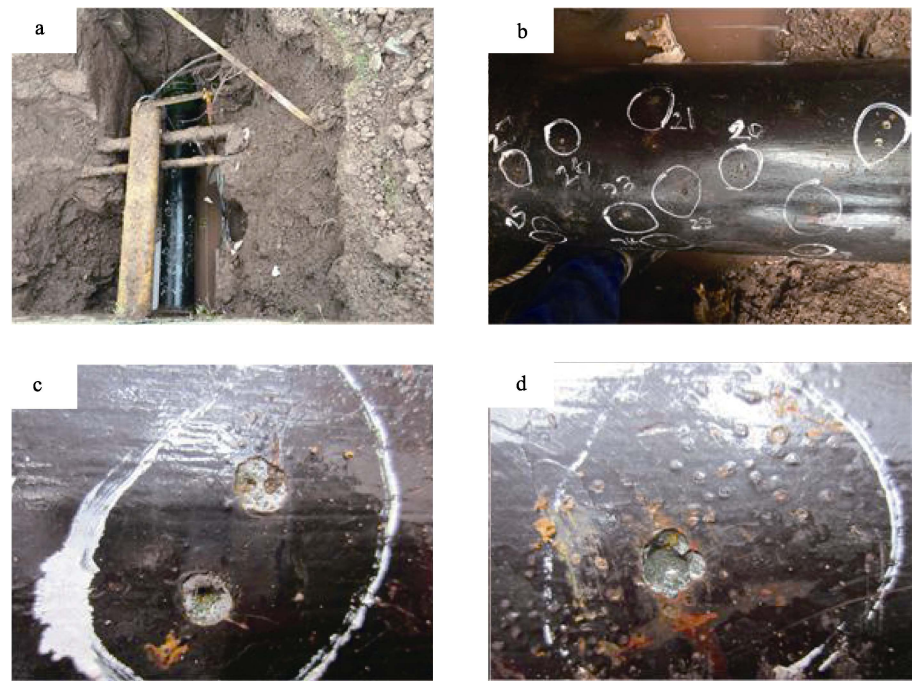
图 2 进站绝缘接头非保护侧管道腐蚀情况 Fig.2 Corrosion of the non-protected side pipeline of the insulation joint entering station
