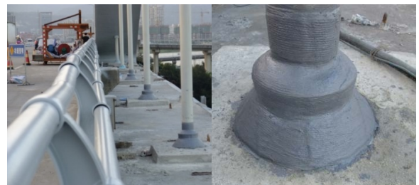
图 6 温州东欧大桥吊杆防水套包覆防腐方案效果 Fig.6 Effect drawing of coating anticorrosion scheme for Suspendor waterproof sleeve of Wenzhou East Europe Bridge
