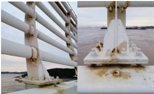
图3 螺栓常规涂层防腐方案 Fig.3 Conventional coating anticorrosion scheme for bolts
