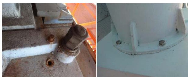
图8 舟山跨海大桥涂装防腐方案腐蚀 Fig.8 Painting anticorrosion scheme and corrosion disease diagram of Zhoushan sea crossing bridge
