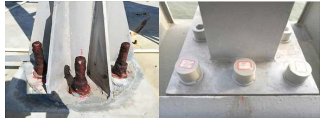
图5 螺栓油性材料和防护盖防腐方案 Fig.5 Anticorrosion scheme for bolt oily materials and protective cover
