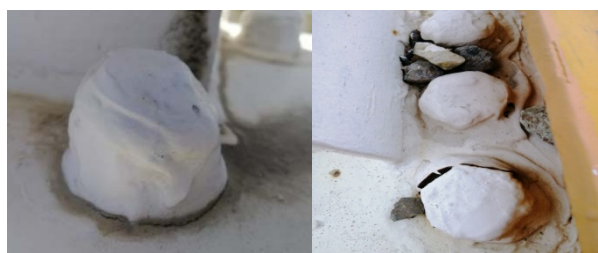
图9 某大桥护栏基座螺栓密封胶防腐方案 Fig.9 Anticorrosion scheme of bolt sealant for guardrail base of a bridge
