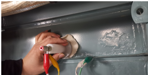
图 10 6 号框附近蒙皮防护涂层起泡区域的电化学阻抗谱测试照片 Fig.10 Electrochemical impedance spectroscopy test of the blistered area of the skin protective coating near frame 6
