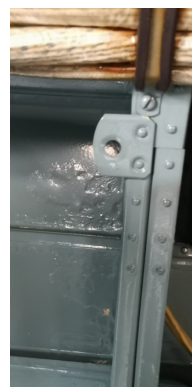
图 4 6 号框与机身蒙皮的连接部位防护涂层起泡的典型外观照片 Fig.4 Typical appearance of protective coating blistering at the connection between frame 6 and fuselage skin
