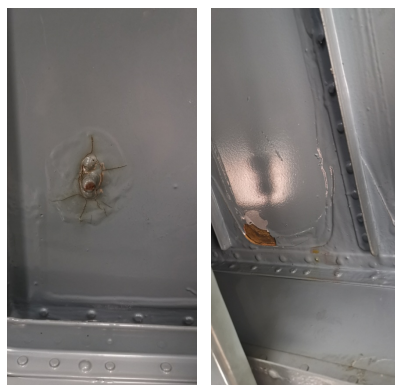
图 3 机身蒙皮与机身外部结构铆钉连接区域防护涂层腐蚀损伤典型外观照片 Fig.3 Typical appearance of corrosion damage of protective coating in rivet connection between fuselage skin and external structure of fuselage
