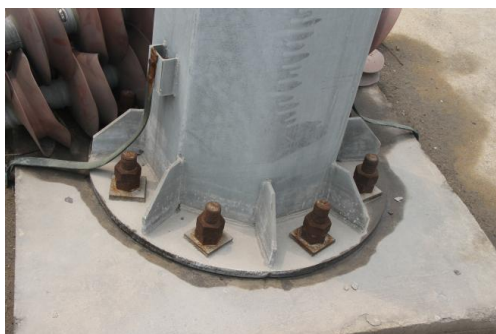
图5 AD 220 kV 变电站避雷针螺栓 Fig.5 Bolt of lightning rod in AD 220 kV substation
