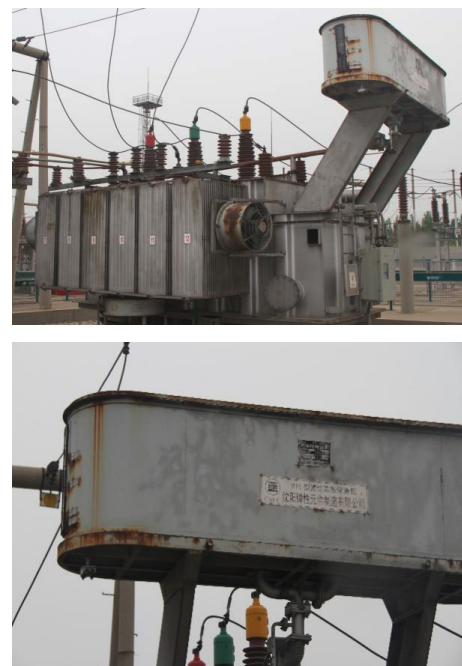
图 3 WD 110 kV 变电站主变压器和油枕 Fig.3 Transformer and oil tank in WD 110 kV substation
