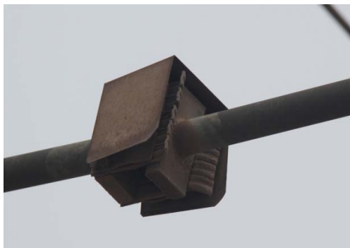
图4 滨州 CK 110 kV 变电站隔离开关 Fig.4 Disconnector in Binzhou CK 110 kV substation
