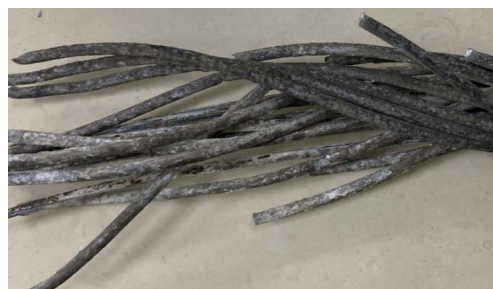
图7 110 kV BS 线退役钢芯铝绞线 Fig.7 Steel-cored aluminium strand decommissioned from 110 kV BS transmission line
